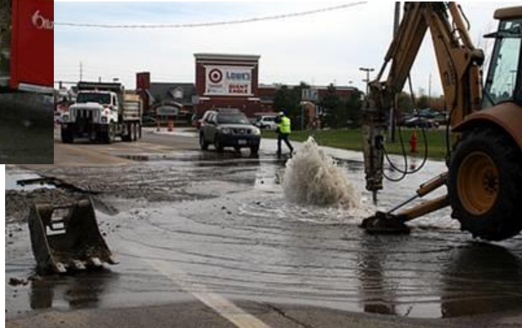
Water Main Breaks
