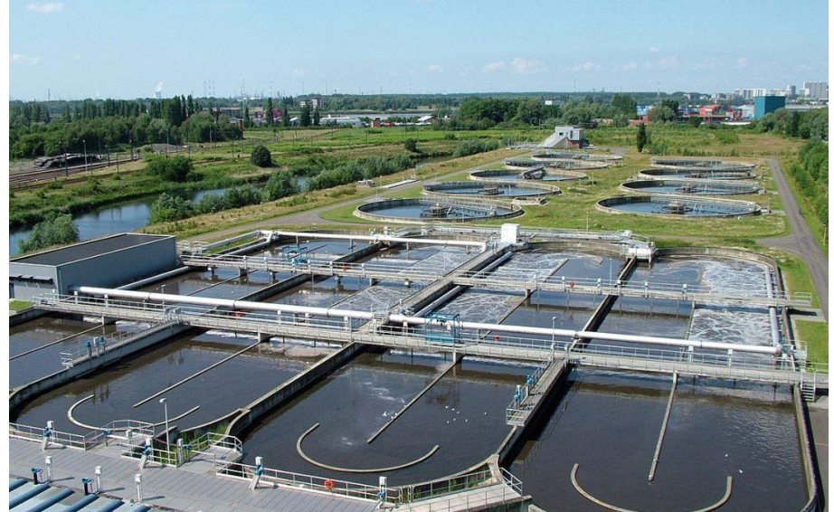
Activated Sludge Plant (also known as a mechanical plant or package plant)
