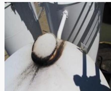
Potential fixed-roof tank defect / leak
